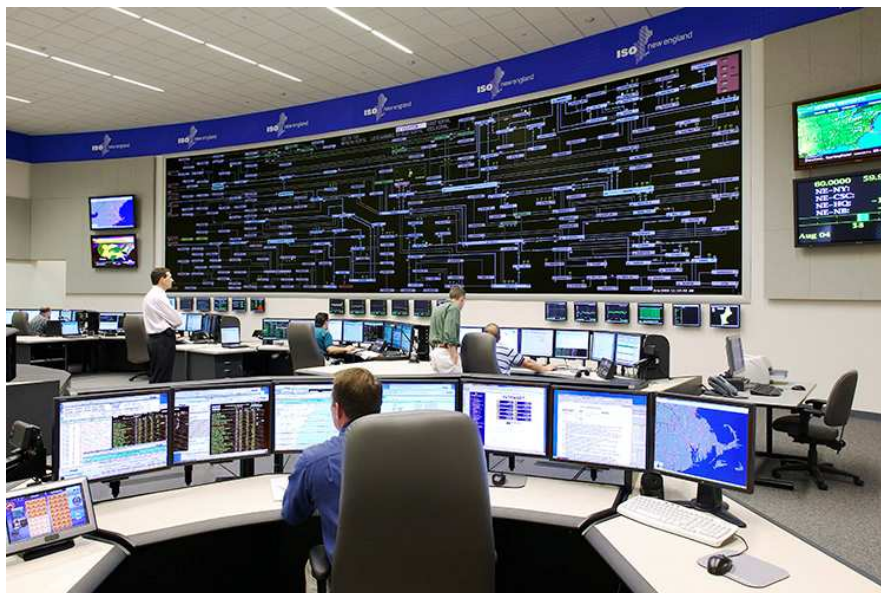
Figure 3. ISO-NE Control Room
