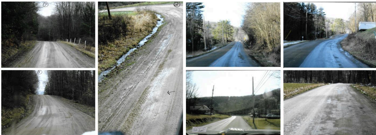
(Photos of road dumping in March and April, 2024)
