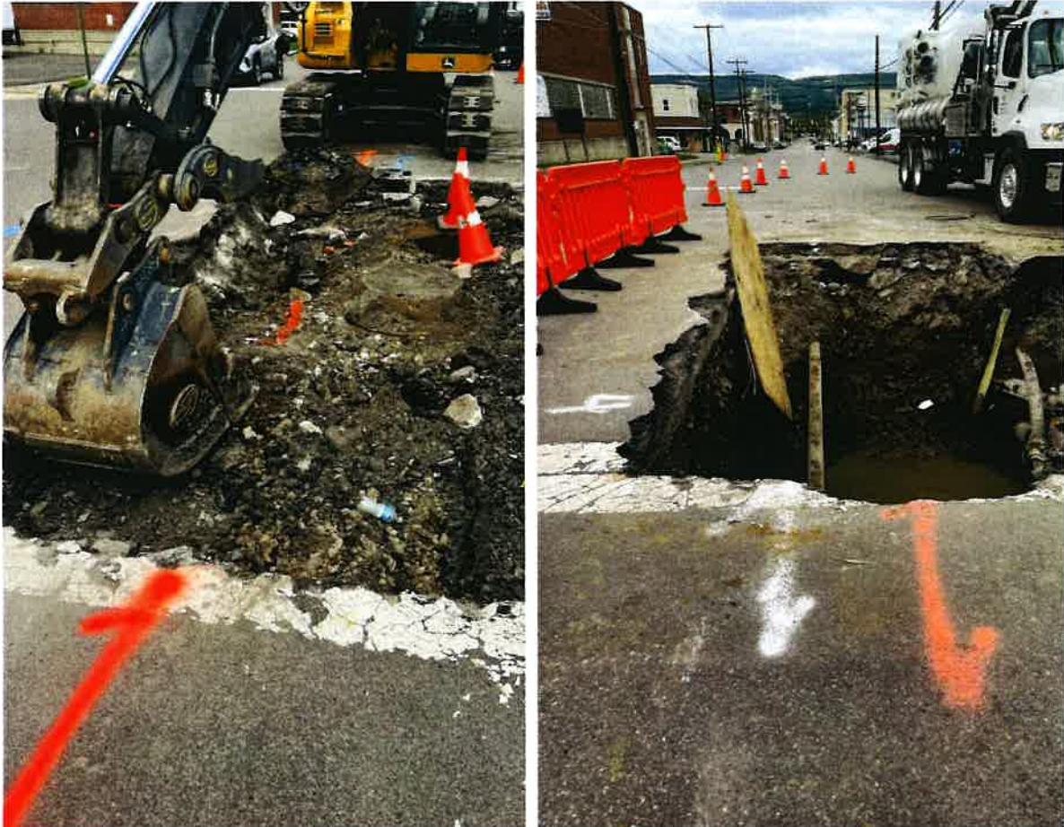
Orange marks placed after renotifying facility owner several times
